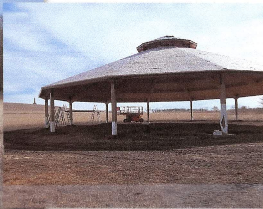
The view from west to east of the dance arbor (under construction). Immediately to the left of the structure is a view of the distant unknown Indian monument. When seated inside the arbor, the monument will be in full view to the east, visually connecting the past to the present.
