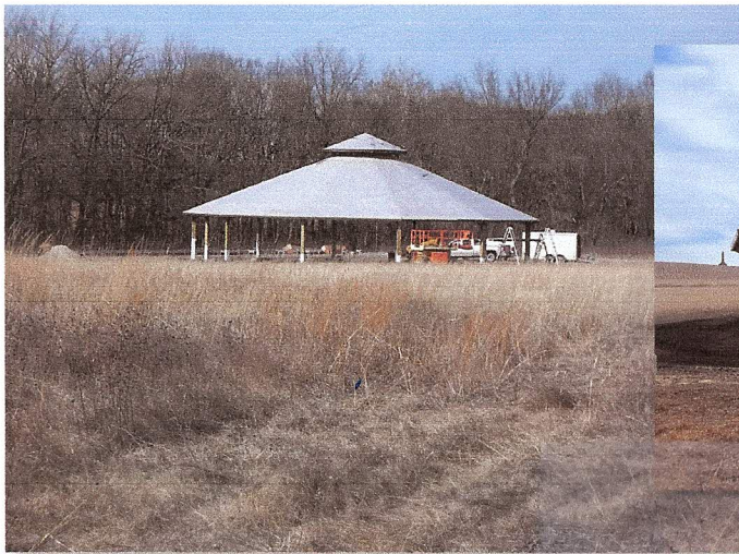
Distant view of the dance arbor under construction. The arbor is tucked down next to the trees, west side of the road that traverses the park north to south. The Kaw Nation plan to hold 3-4 dances a year under the arbor.
